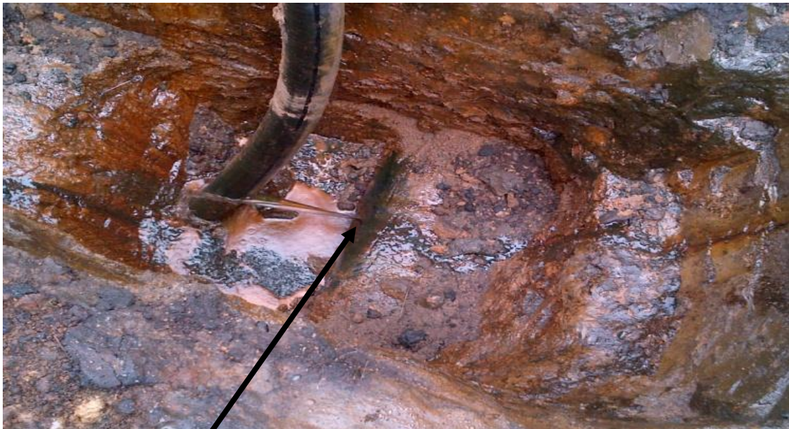
Hacksaw cut at 9 O'clock position on pipeline
